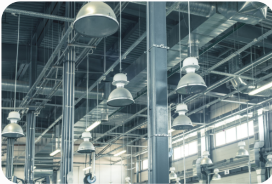
High-bay factory lighting setup ensuring uniform working plane illumination.
